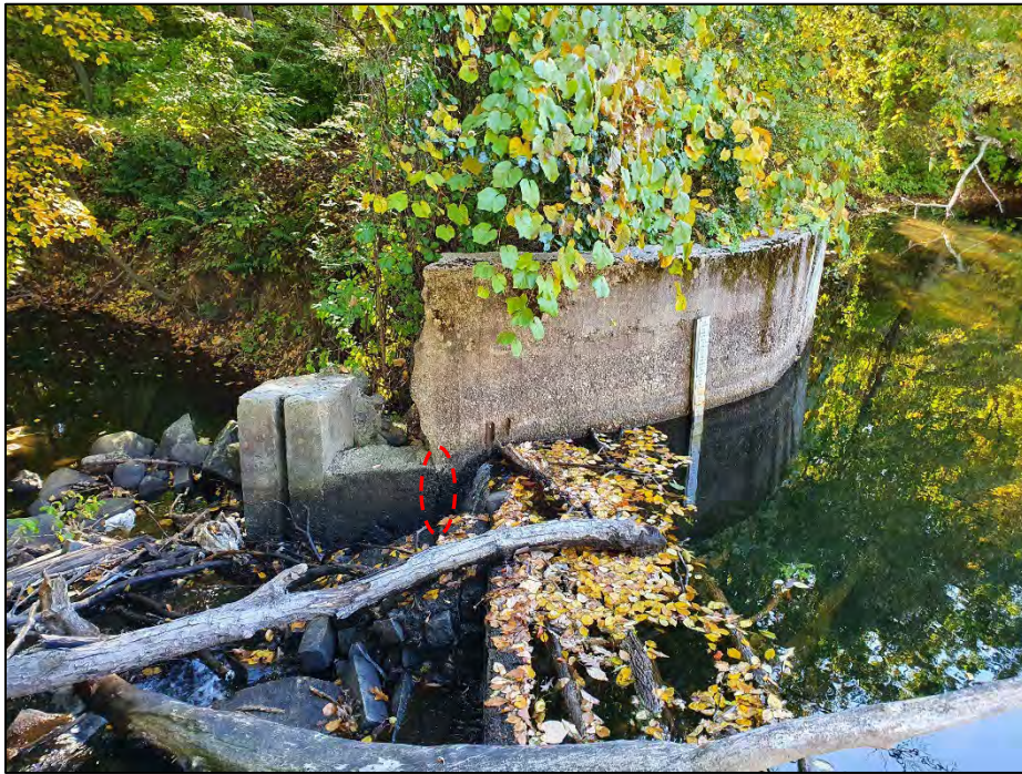
Photo No. 17.: Overview of the right upstream wall from the spillway channel looking right. Note the crack along the downstream section.
