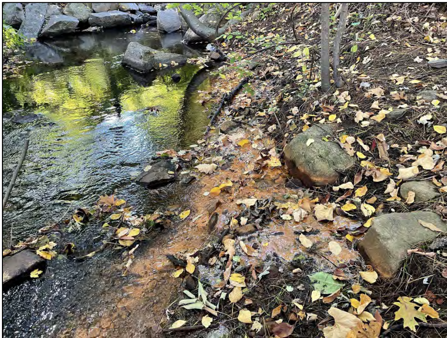
Photo No. 20.: Observed seepages with iron oxide flocculant approximately 15 feet downstream of the downstream channel left wall.
