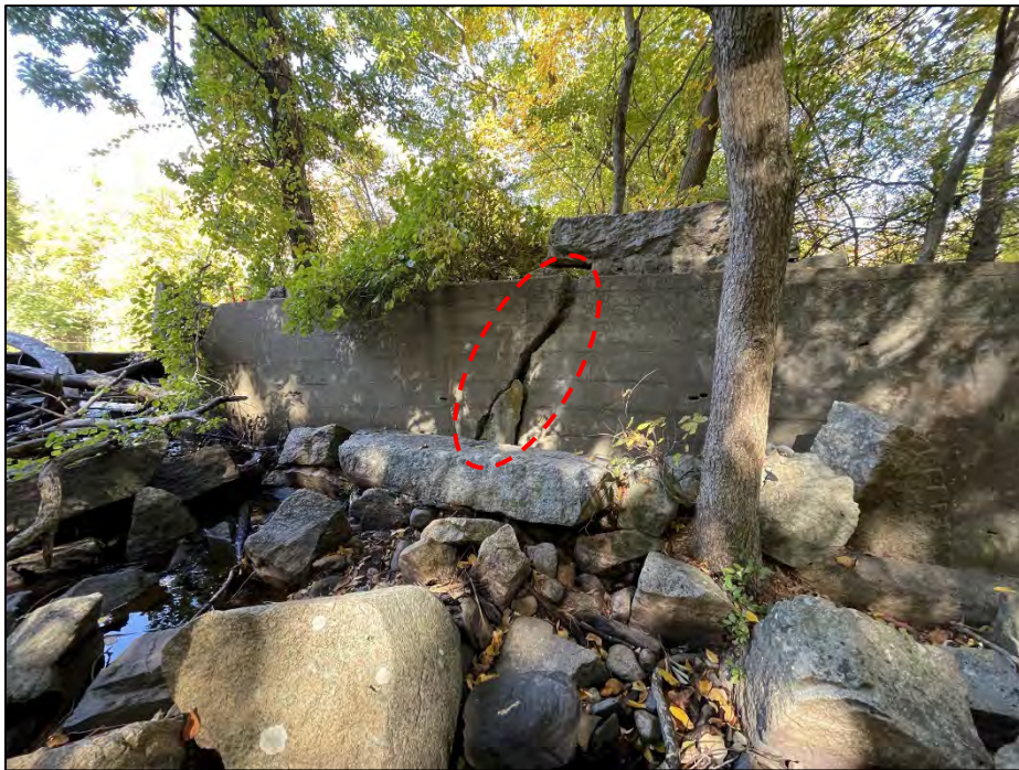
Photo No. 16.: Concrete wall left of the spillway. Note the 5-inch crack.
