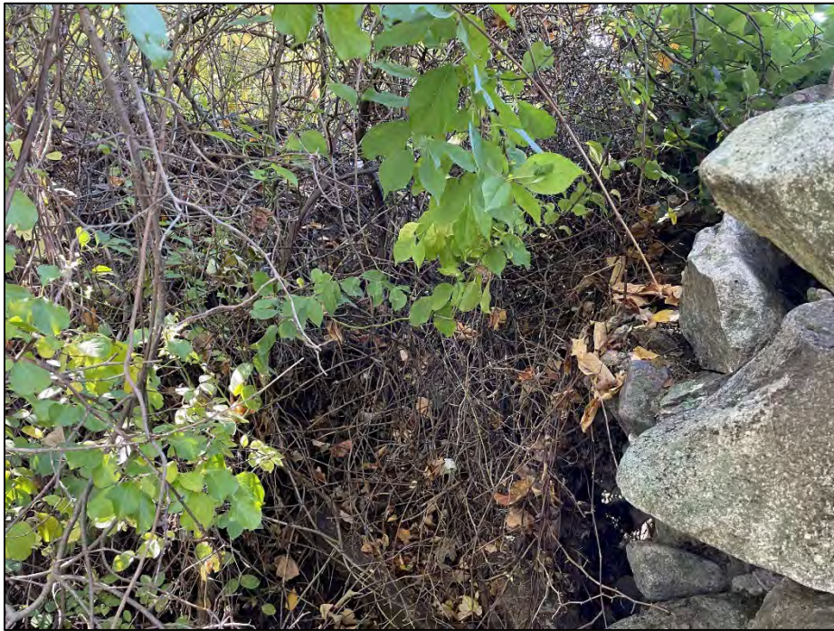
Photo No. 19.: Eroded area behind the right upstream wall.
