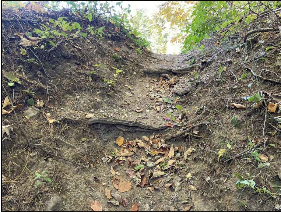
Photo No. 13.: Erosion path from the crest to downstream toe near Sta. 1+00.
