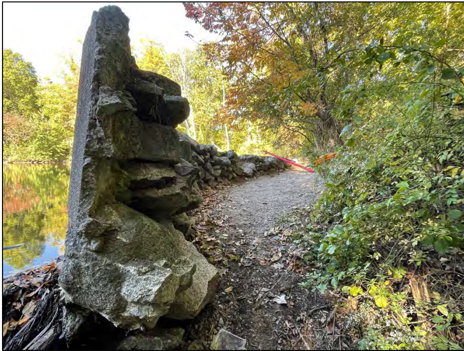
Photo No. 9.: Erosion of the dam crest immediately behind the upstream wall left of the spillway.
