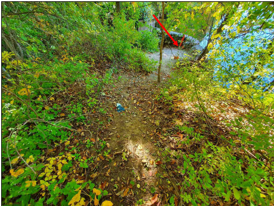
Photo No. 8.: Crest from near Sta. 1+10 looking right. Note erosion of the crest behind the upstream wall left of the spillway (arrow).
